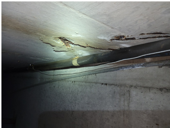
Photograph #5 – Spalling and slab damage
